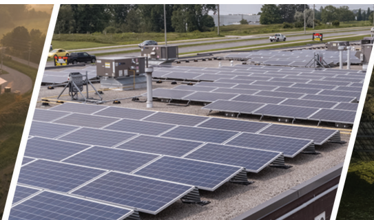
125kW Flat Roof FIT 2
