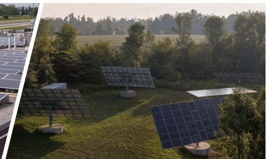
50kW Net Metering Dual Axis Trackers
